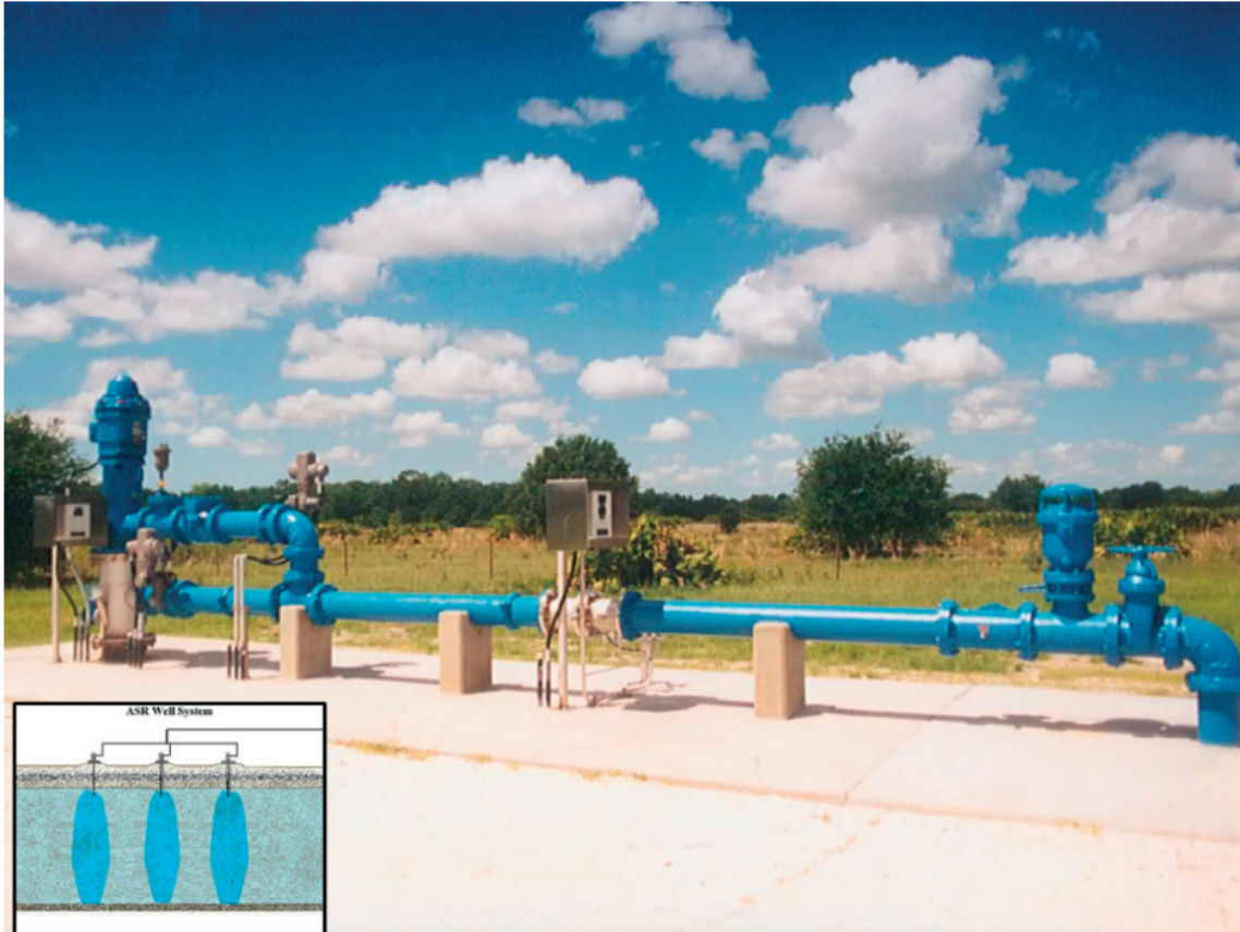
Figure Box 1. Aquifer Storage and Recovery (ASR) system example in Southwest Florida with a capacity of 30 million M3 consisting of 21 wells.
